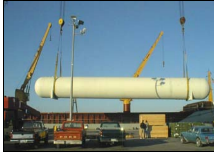
LOADING TANK WITH SHOREGEAR
